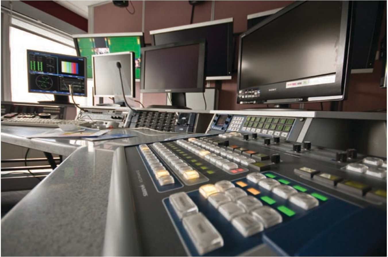
A look at the new master control room reveals Harris master control switchers, control panels and on-screen monitors.
