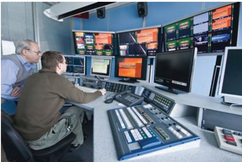
Czech TV master control room personnel use Harris Videotek multiformat monitors to track and measure HD-SDI signals.
