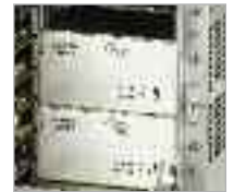
Backup Power Supplies
